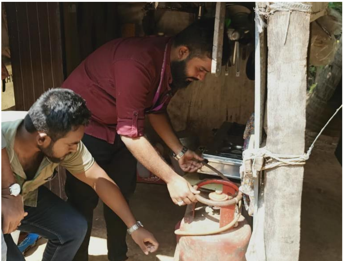
MEMBERS OF OUR CITIZEN CONSUMER CLUB EXAMINING THE CONDITION OF RUBBER PIPE OF CYLINDER IN ONE OF THE HOUSE
