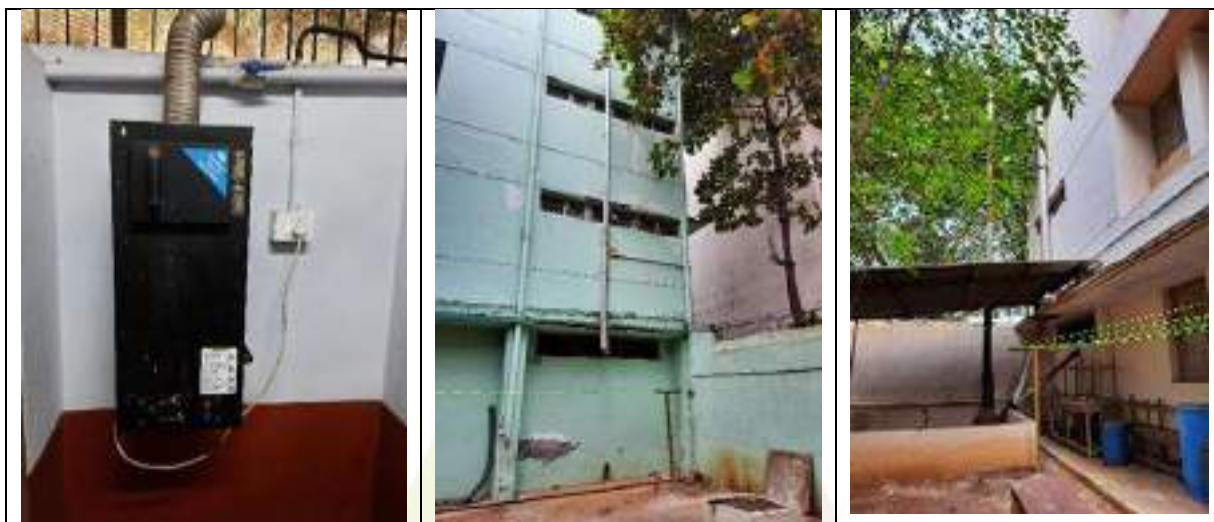
Incinerators arrangements at women's hostel
