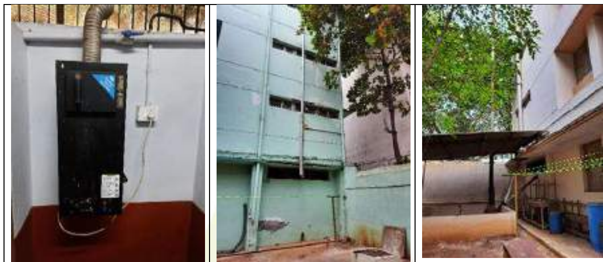
Incinerators arrangements at women's hostel
