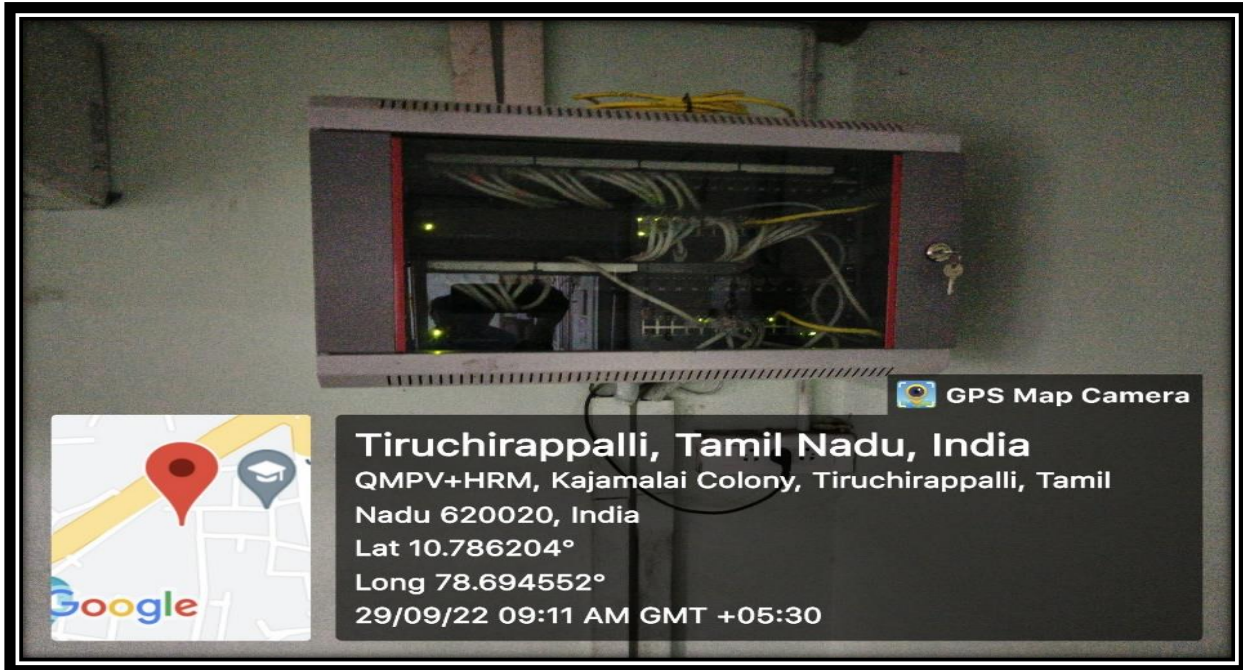
NETWORK SWITCHES IN DEPARTMENT OF COMPUTER SCIENCE
