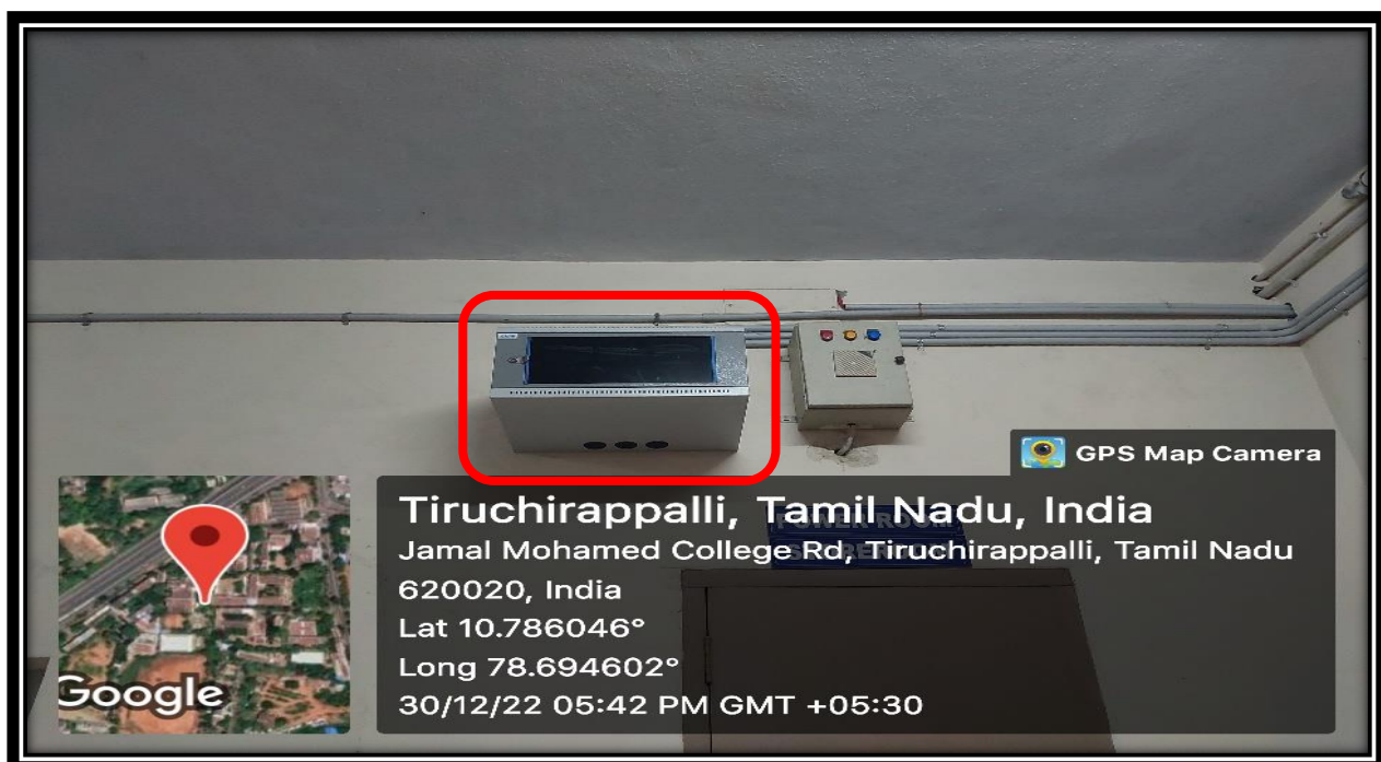
NETWORK SWITCHES IN IT-BLOCK
